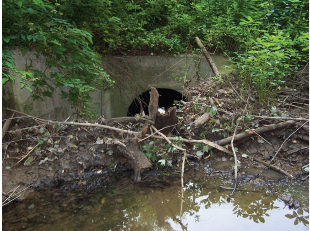
Figure P.3.25 Debris and Sediment Buildup
